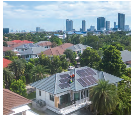
Green, competitive, and inclusive cities. Solar panel installation at Grand Bangkok Boulevard, Thailand. GMS-2030 aims to improve disaster and climate change resilience .
