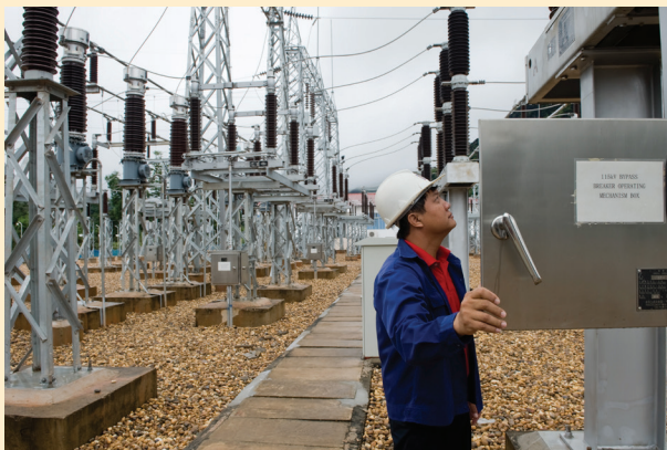
An engineer at the Nam Theun 2 Hydropower Project. Routine inspection at a high-voltage cross-border substation ensures safe and reliable electricity flow between Lao PDR and Thailand.
